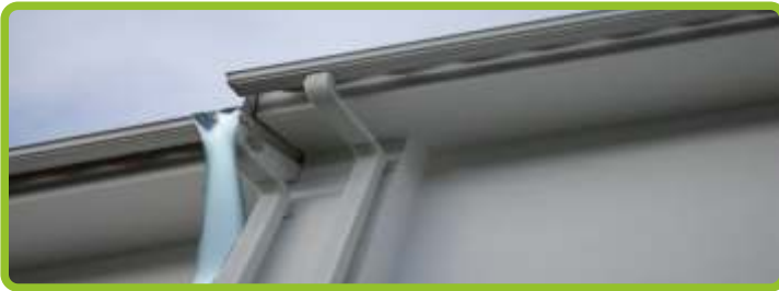
Example of an undersized gutter.
